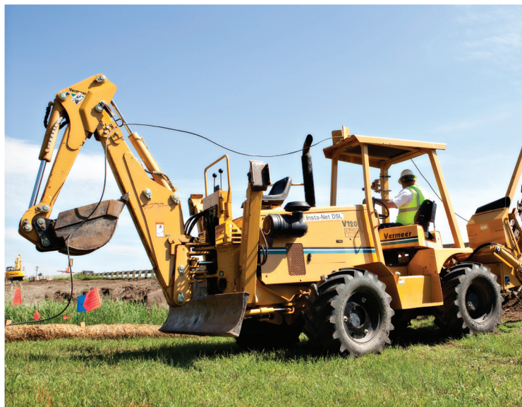
RTC prepares to place fiber in the ground to connect customers such as BakkenLink Pipeline.
